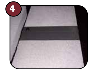
Silicate sealer has been removed on bottom portion of masking tape.
