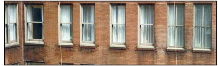
A competitor's unsuccessful test patches on the Fairmont Hotel in New Orleans, LA.
